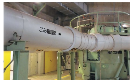
廃棄物空気輸送管 Pneumatic trash-carrying ducts
